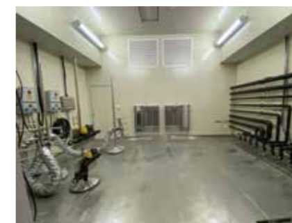
R290 A/W heat pump performance lab
