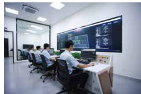
Digital central control room
