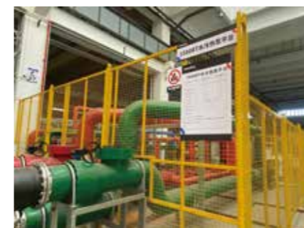
1500RT water cooled heat pump platform
