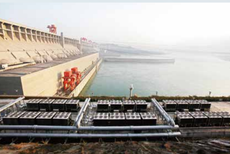
◀ Three Gorges Hydropower Project Location: Yangtze River, China Product: Air-cooled&water-cooled screw chillers, AHU
